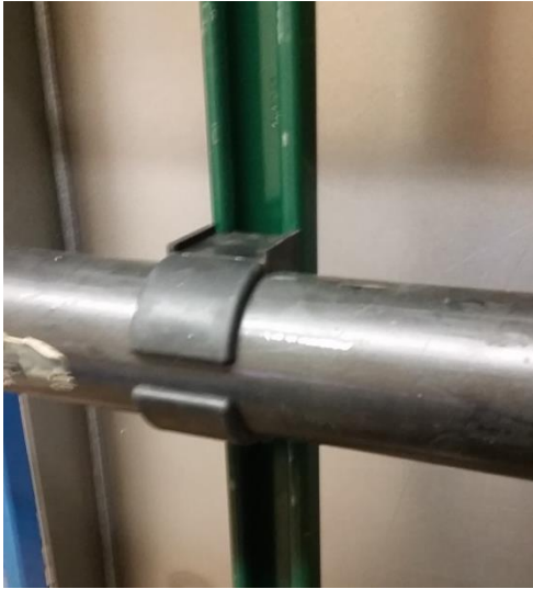
Figure 14: Pipe Stand Isolation Rubber
